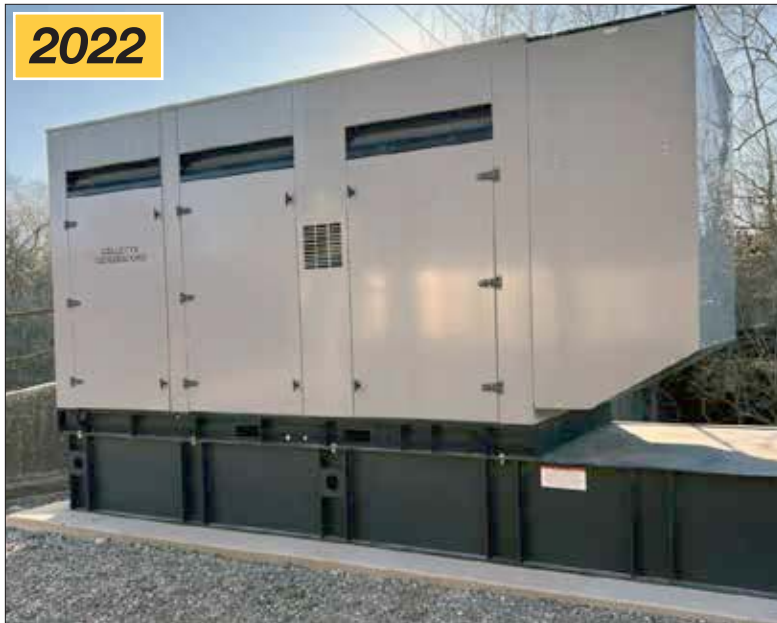
Gillette SPVD-6000-3-4-2, 660-kW Diesel Generator
