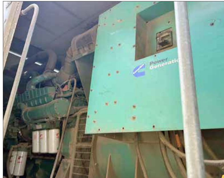
Cummins DFGE 5693579 750 KW Diesel Generator
