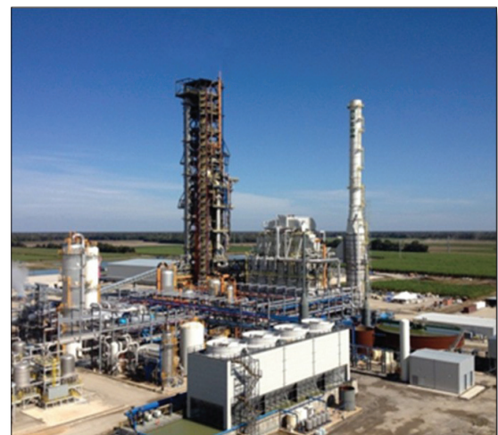
Fig 9 Nucor Steel Louisiana DR plant with CO 2 absorption and sulphur removal system
