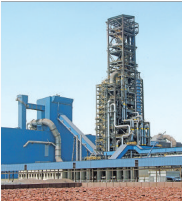
Fig 1 AUMUND 250tph hot DRI conveyor, Hadeed, Saudi Arabia
