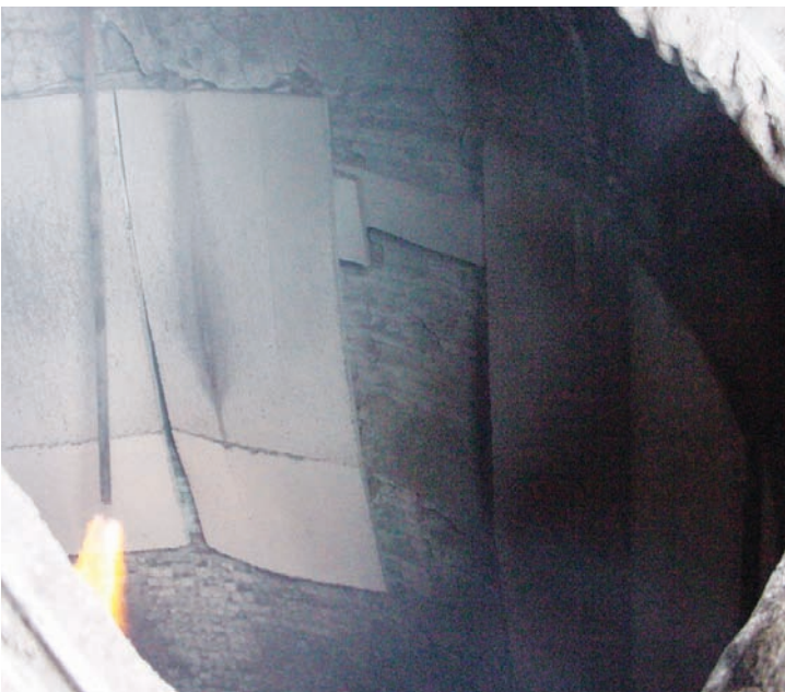
ⓐ Fig.9 Severe distortion to throat armour
