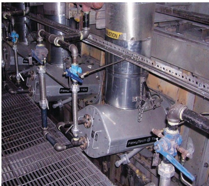
Fig.7 TSX burners at Rocky Mountain
