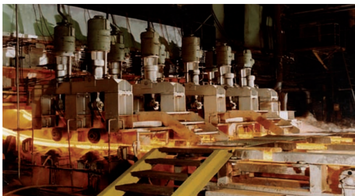
ⓐ Fig.3 Straightening unit at CCM 1
