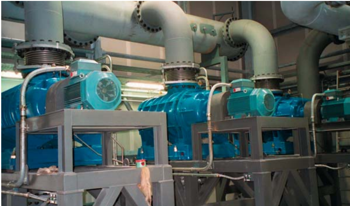
© Fig.1 40 ton steel degassing system – first stage dry mechanical booster pumps
