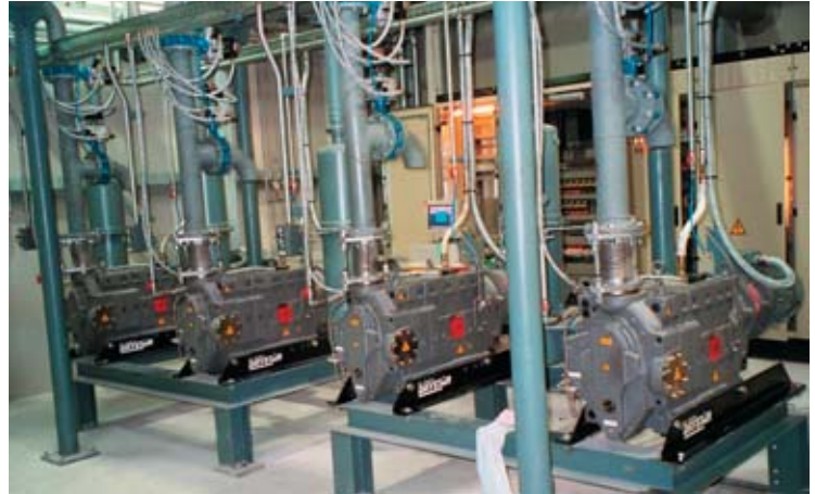
Ⓐ Fig.3 40 ton steel degassing system – dry claw primary pumps
