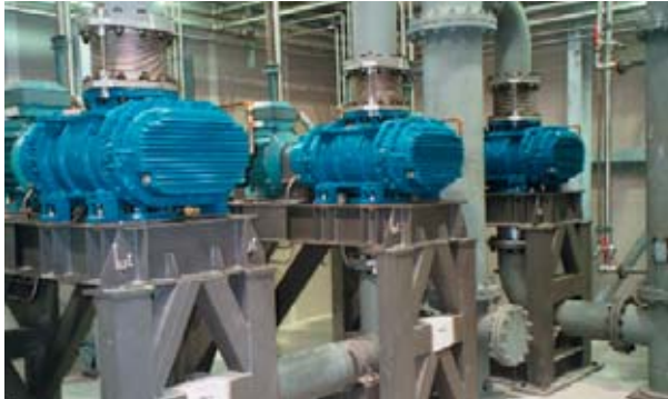
Ⓐ Fig.2 40 ton steel degassing system – inter stage dry mechanical booster pumps with heat exchangers
