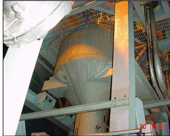
● Figure 5 Reactor vessel
