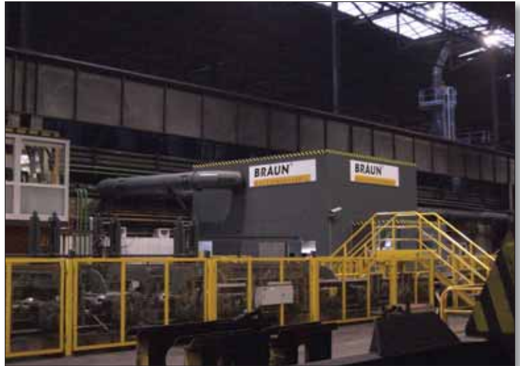
Ⓐ Fig 5 HP grinding machine at SAARSTAHL, Neunkirchen, Germany (grinding machine encapsulated by grinding cabin and connected to dust extraction system)
