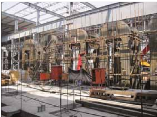
Ⓐ Fig 2c installation of the cold-rolling tandem mill
