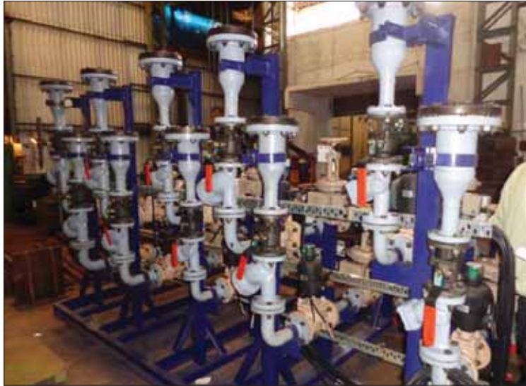
Fig 5 New Air valve skid for air supply of segments 1 and 2
