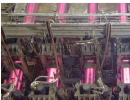
Fig 7 Top view on straightener during hot commissioning of strand 1 (right)
