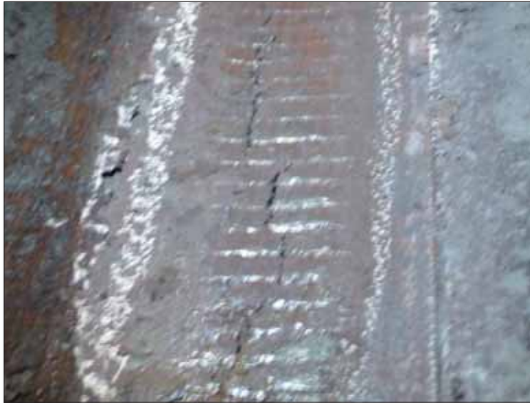
Fig 1 Web surface cracks on beam blank
