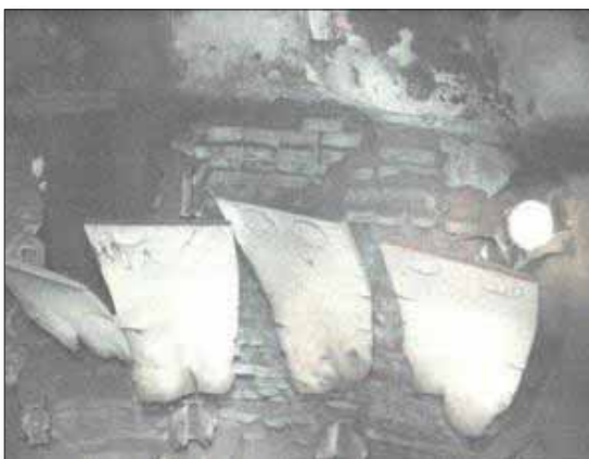
Ⓐ Fig 12 Severely damaged throat armour
