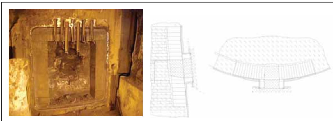
Fig 9 Campaign extension repairs to the taphole
