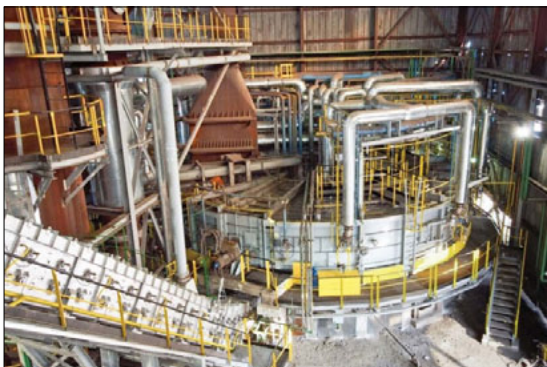
Fig 5 Rotary hearth furnace of RedIron recycling plant
