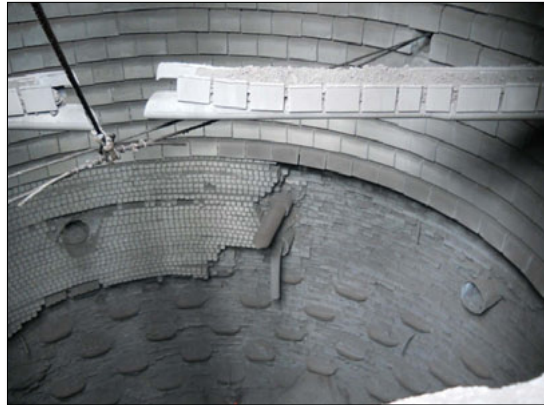
Fig 10 Collapse of lining in upper stack
